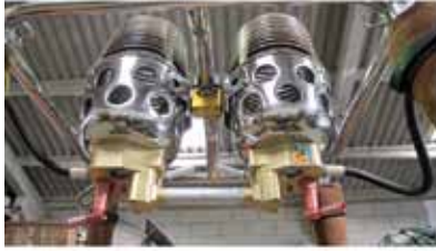
Double Burner Unit
