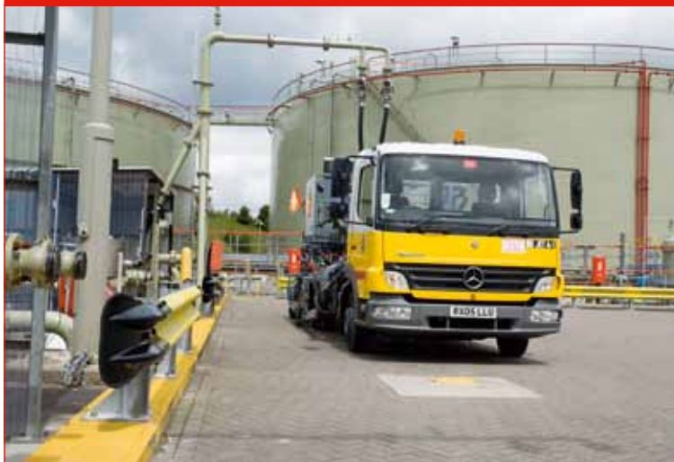
Picture 17: Fuel farm at Gatwick Airport
